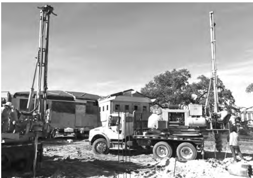
Construction crews move “Norcliff” or the Norwood House as a new foundation is prepared.
