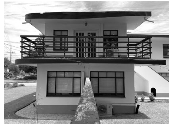
Sagging eaves will be structurally reinforced this year.
